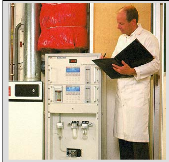
An ADC gas analyser in use at a boiler facility
